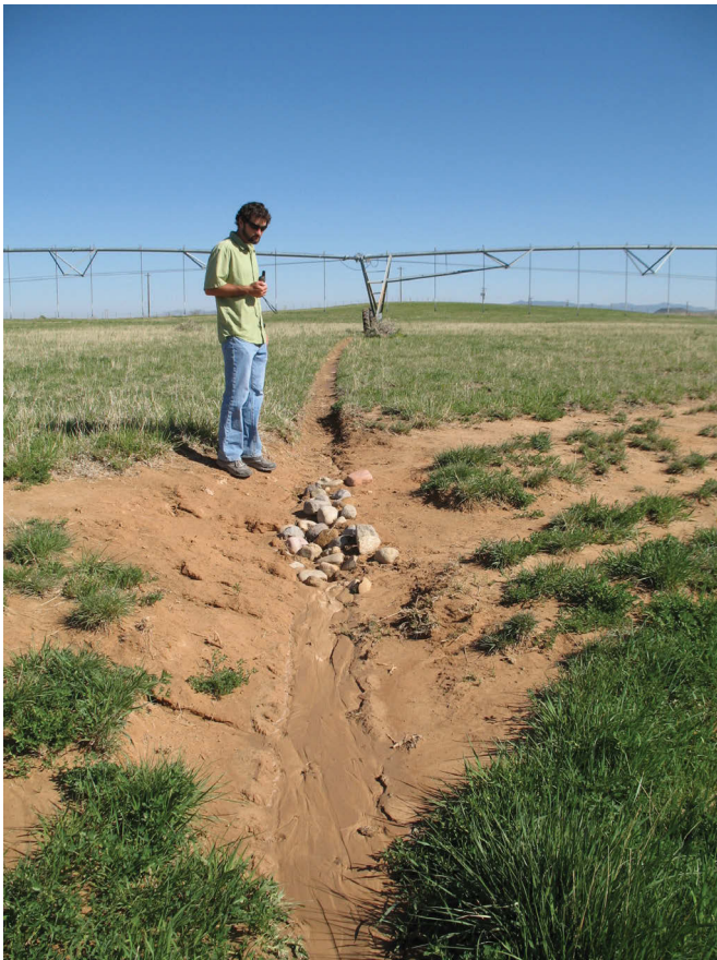
Figure 28. Repair to irrigation pivot track where it crosses the scarp of the EGWF1 fissure (view is to the northwest). Photo taken in May 2009.
